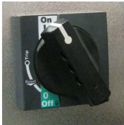
Image 2-2 – Main Disconnect switch
