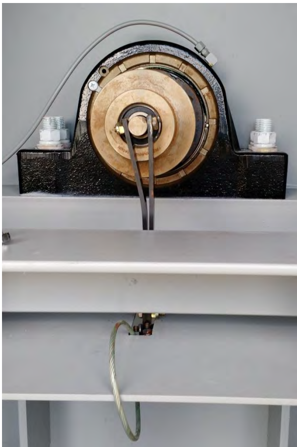
Image 3-8 – Backspin preventer installed
