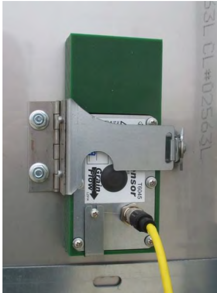
Image 20 – Incoming moisture sensor
