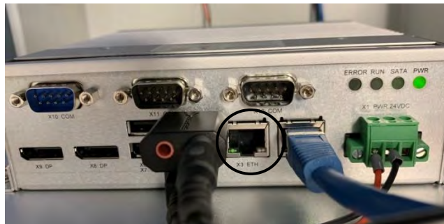
X3 Ethernet port (circled) in touch panel box
