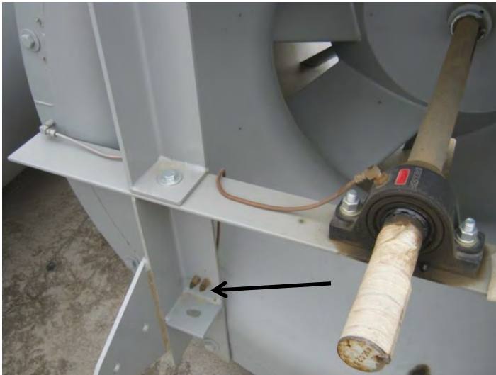
Image 3- 4 – Grease zerks for blower shaft bearings
