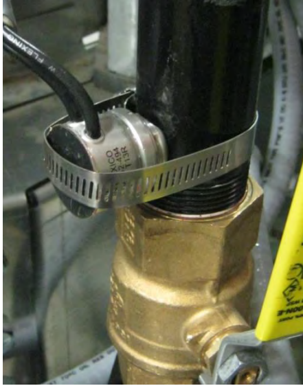
Image 4-4 – Vapor over-temp switch
