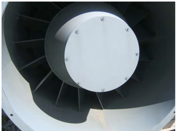
Image 3-9 – Shaft cover plate on top of blower
