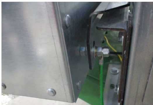
Grounding at main power box
