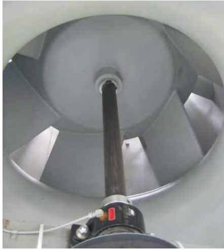
Image 15 – Blower, drive shaft
